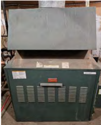
Figure 30 - DHW Boiler (B-3)
