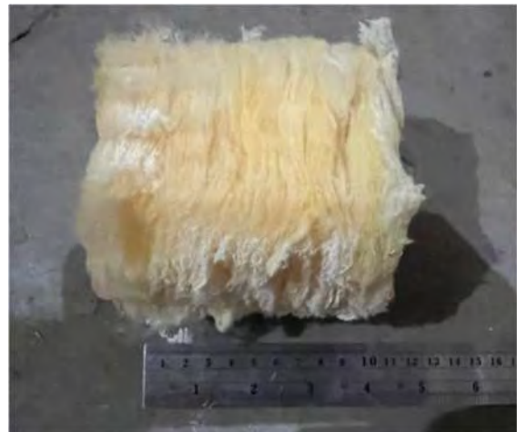
Figure 13 – 3.5" Batt insulation in Boiler Room
