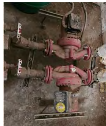
Figure 35 - Space Heating Circulation Pumps (P-3,4)
