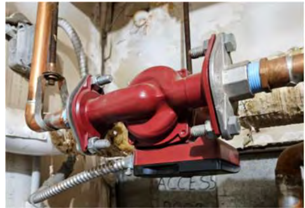
Figure 33 - DHW Recirculation Pump (P-7)
