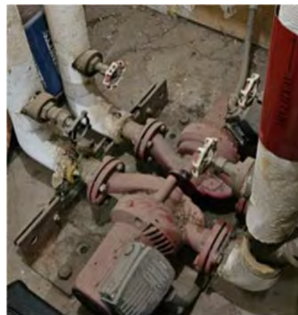
Figure 29 - Space Heating Circulation Pumps (P-1,2)
