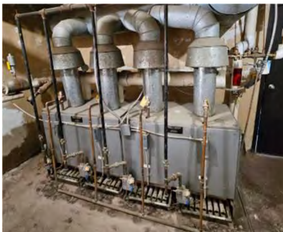
Figure 28 - Space Heating Boiler Plant (B-1)
