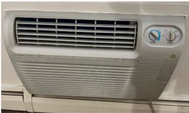
Figure 40 - Original In-Unit PTAC
