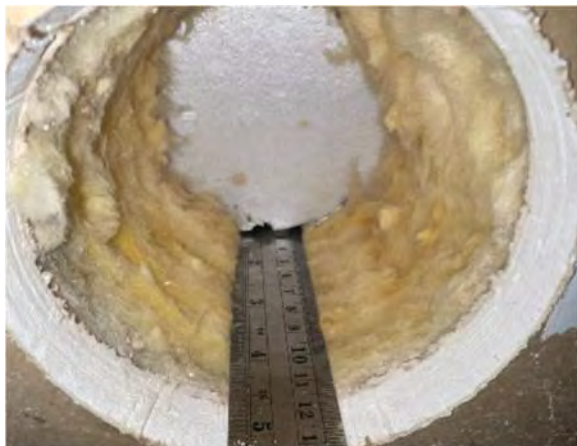
Figure 12 – 3.5" depth batt insulation and 1" expanded polystyrene in Boiler Room
