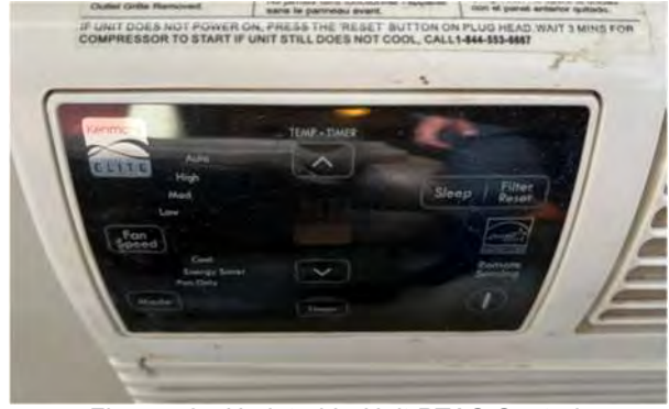
Figure 43 - Updated In-Unit PTAC Controls
