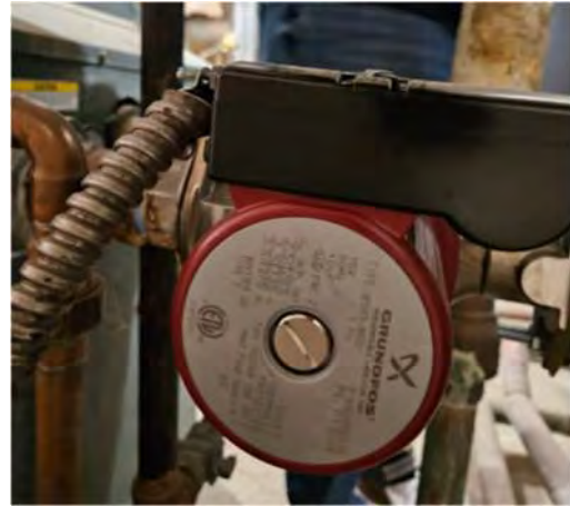
Figure 31 - DHW Circulation Pump (P-5)
