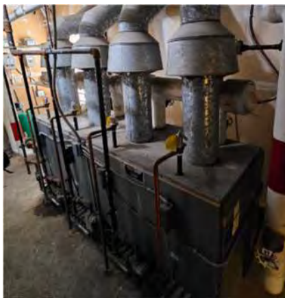
Figure 34 - Space Heating Boiler Plant (B-2)
