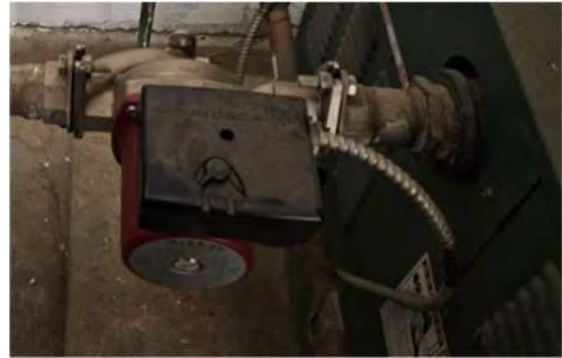
Figure 37 - DHW Circulation Pump (P-6)
