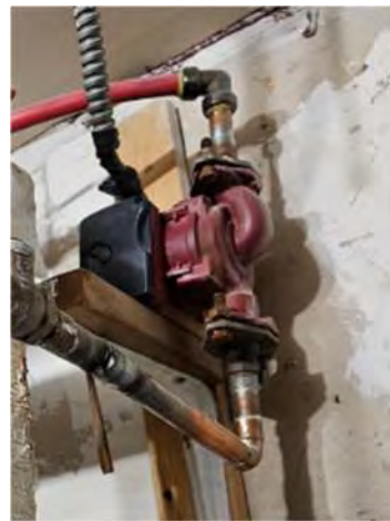
Figure 39 - DHW Recirculation Pump (P-8)
