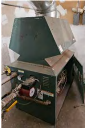
Figure 36 - DHW Boiler (B-4)
