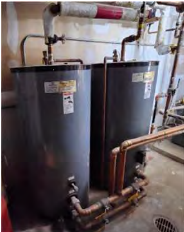
Figure 38 - DHW Storage Tanks (ST-3,4)
