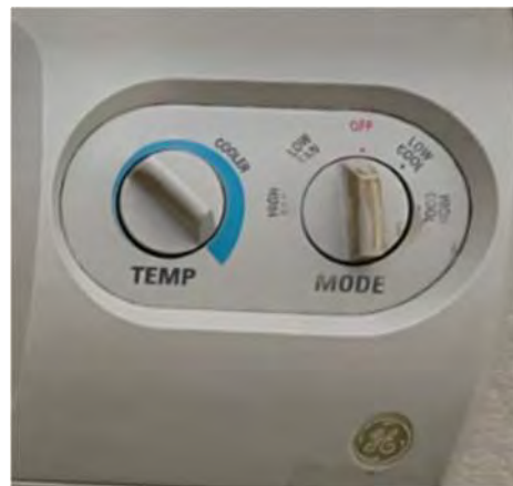
Figure 41 - Typical In-Unit PTAC Controls
