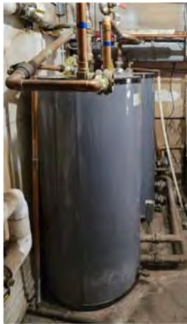
Figure 32 - DHW Storage Tanks (ST-1,2)
