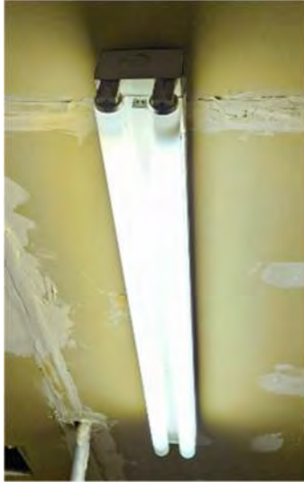
Figure 16 – Fluorescent Ceiling Mount Strip (T12-2)
