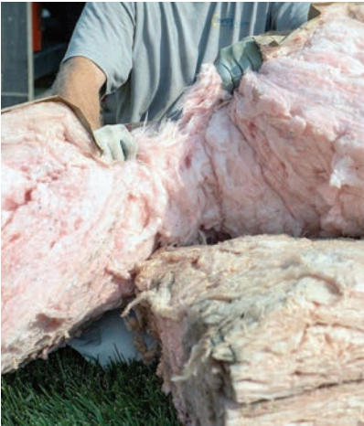
This home in Conifer needed multiple energy upgrades, including attic, floor, wall and duct insulation.
